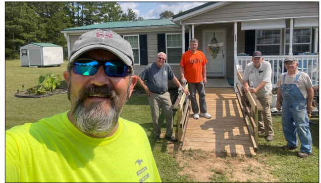
Rebuilding Hope volunteers (from left) Tom Wille, Dave Burns, Walt Slaton, Randolph Wilson and team leader Cliff McClanahan built this ramp for a resident in Vance County.
