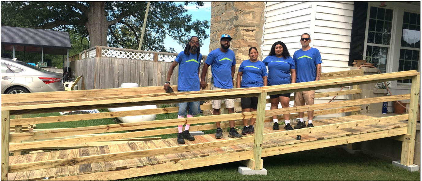
This Clayton Homes employee team helped build this wheelchair ramp in August at a home near Satterwhite Point.
