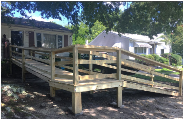
A Clayton Homes employee team helped build this ramp in July in Henderson.
