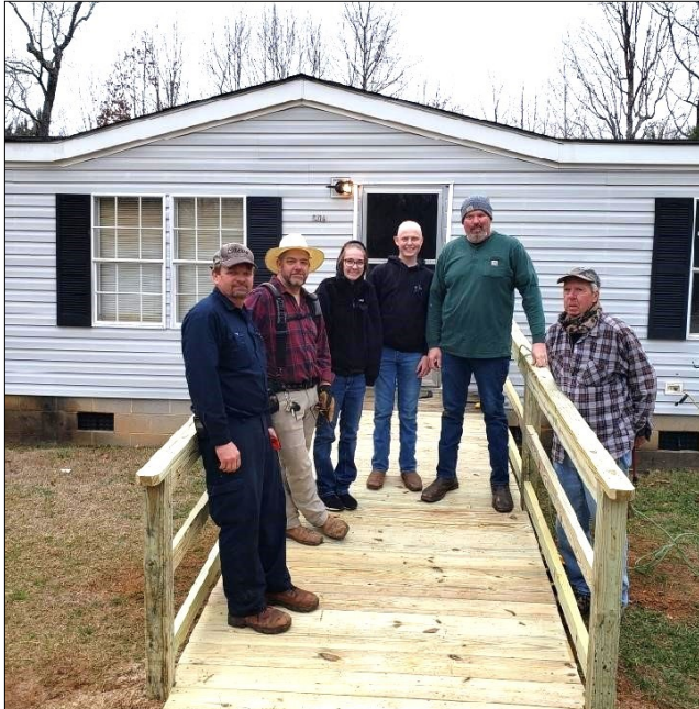
Members of South Henderson Church of God partnered with Rebuilding Hope to build this ramp in Henderson in February. Pictured are (from left) Ray Patrick, Wayne Burnette, Haleigh Burnette, Jackson Gordon, Brandon Gordon and Roy Munn. April Burnette took the picture.
