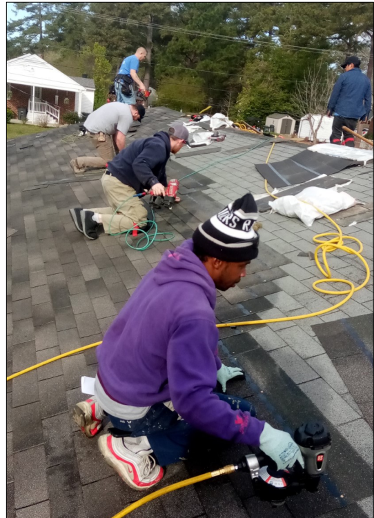
Five employees of Clayton Homes of Nashville partnered with Rebuilding Hope to replace this roof in Rocky Mount. The employees participated as part of the company's Volunteer Time Off program.
