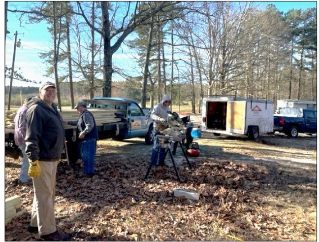
A crew at work on one of the 40 ramps volunteers have built since the year began.
