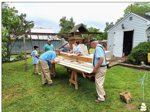
The SOS Facia Fixers team — whose ages ranged from 13 to 91 — installed siding on this home in Warrenton.
