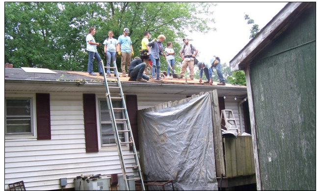
SOS Ladder Leapers team replace this roof on Glover Street in Henderson. It was one of five roofs replaced by the 2023 campers.
