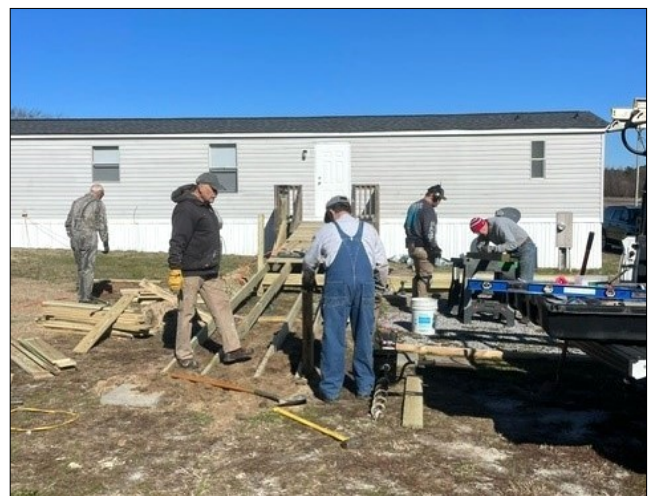
RHI volunteers assist members of Central Baptist Church as they build a ramp.
