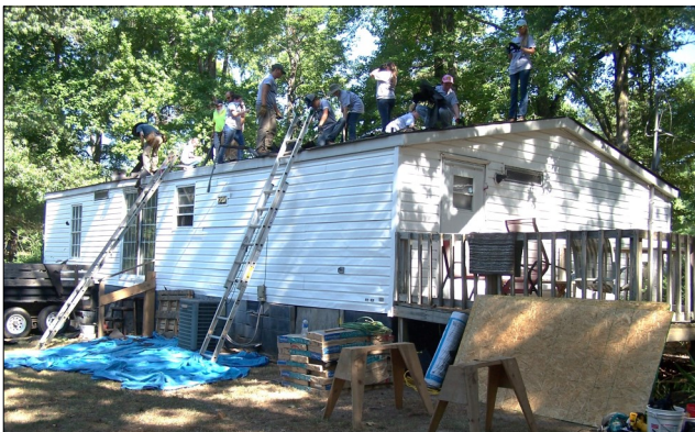
Servants on Site tackled six roof jobs during their week of work. Three were in Vance County and two in Warren County by the Jigsaw Jammers and Nail Gunners teams and one in Granville by the Fascia Fixers team. The job above by the Drip Edgers team is in the Deerfield Run area.
