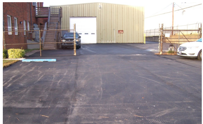
Photos in this column show the repaved areas at the front and rear of the building. More photos, next page.
