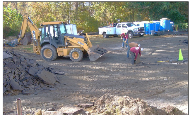
Between the Before and After: Tons of old pavement are removed before paving can begin.
